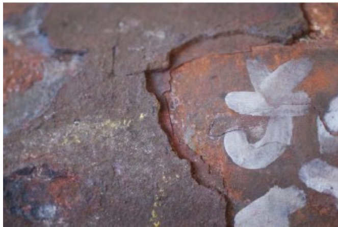
Figure 4: Thick oxide scale on outside of pipes of both refinery convection sections indicating overheating.
