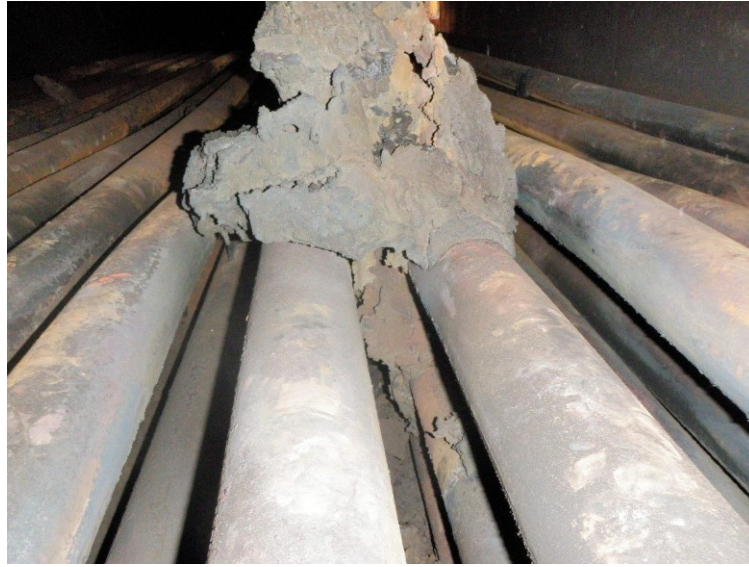
Figure 2: Burst convection section (shock tube) pipe in 12 o'clock position with burnt residue covering the rupture
