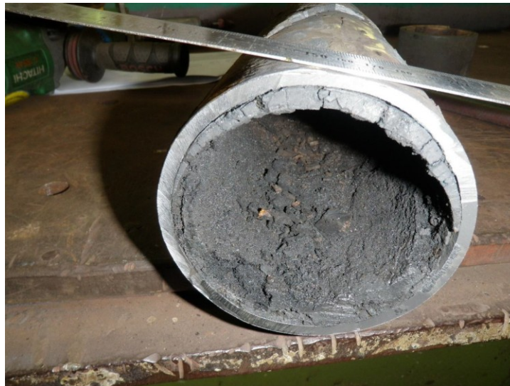
Figure 5: Extensive internal coking in 12 o'clock position (highest heat flux)
